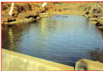
Picture of the Karoli Check Dam at Mokhada-Jawahar in the summer of 2010. This check dam was completed by Impact India Foundation - supported by the Rotary Club of Mumbai-Borivali (E) and has benefitted about 1000 villagers.
