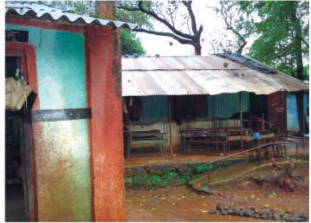
Mendwan Ashramshala with leaking and rusted tin roofs
