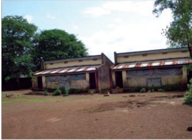
Embur Ashramshala in a dilapidated condition
