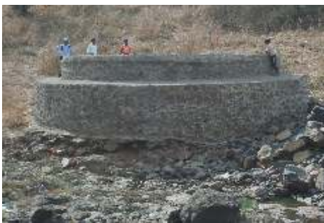
The well in Jambulpada in need of repair
